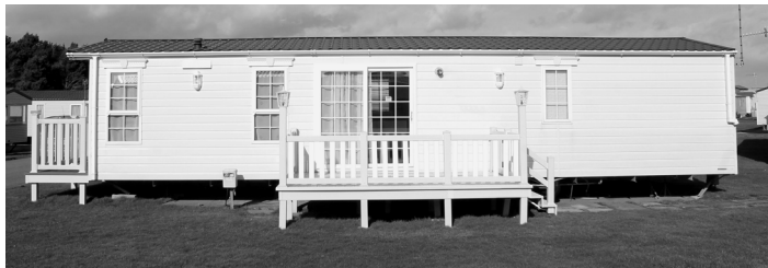
Does not meet standard for skirting.
